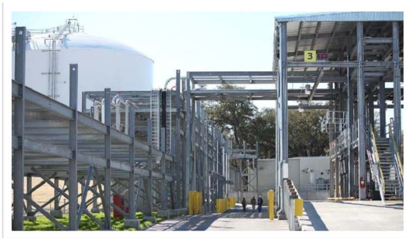
The terminal in Charleston, USA is now fully operational
